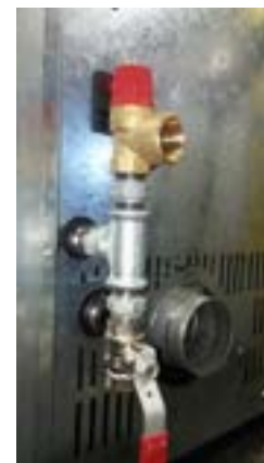
Connection of pressure relief valve and 3 bar safety valve.
